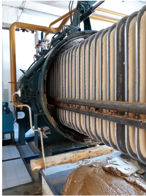
Figure 2. Horizontal pressure leaf filter (Amafilter BV, Alkmaar, The Netherlands; surface: 60 m 2 ) used in the industrial winterization process.
